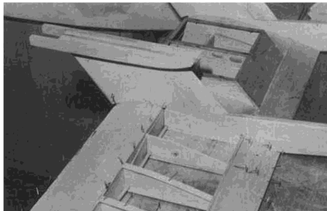
Sealander II center section during construction. Note aileron control tubing in place. Wing is semi-symmetrical but built on flat surface.
