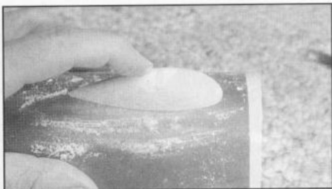
RIGHT: Fuel cap fairing is fitted to hatch by rubbing on sandpaper, grit side up.
