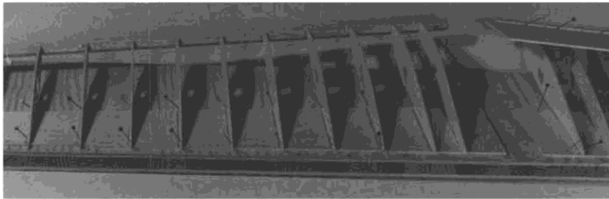
Start of wing construction. Wings are built upside down. Balsa sheet pinned to the board is top t.e. sheet.
